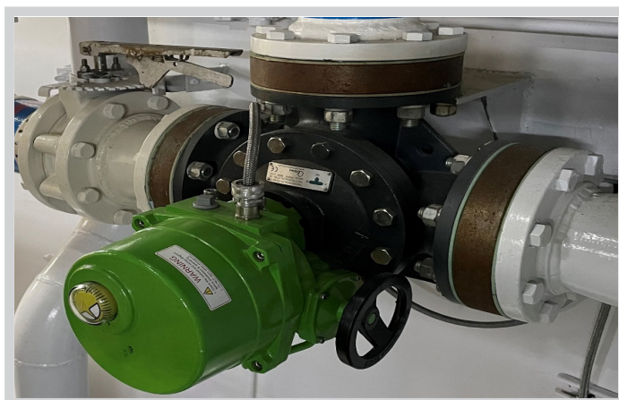
Installation of 3 way control valve GFMT with machined spacers and CAR-H actuator.
