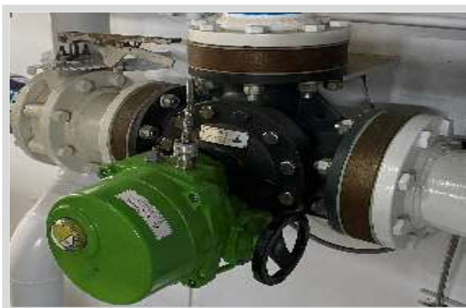
Installation of 3 way control valve GFMT with machined spacers and CAR-H actuator.
